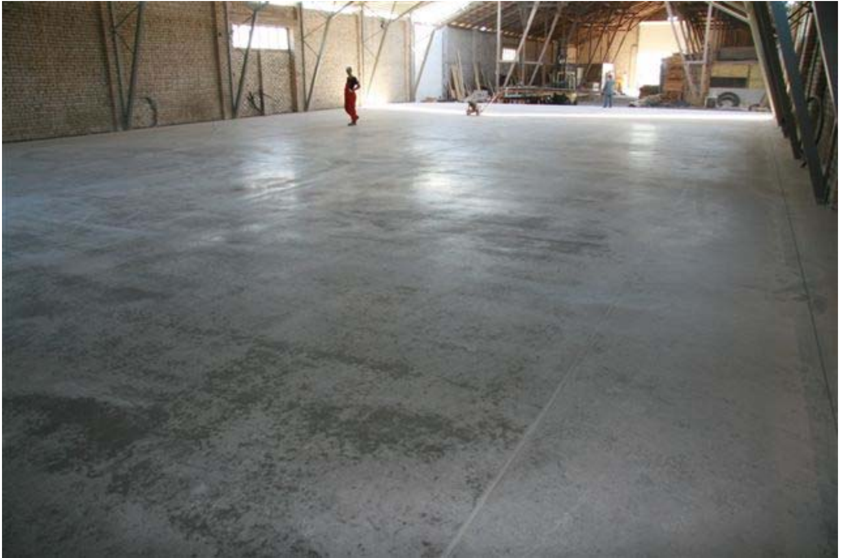
WAREHOUSE FLOOR shown before polishing. Not one shrinkage crack was found after inspection. For the first time in their practice workers started to polish the floor without preliminary patching. Reflection of natural light from bare concrete is already there.
